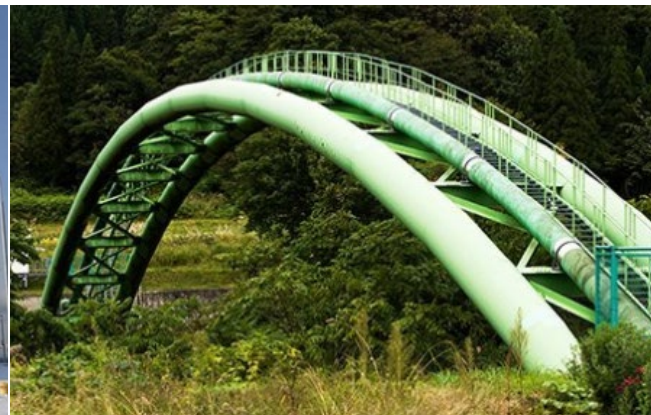
Natural Gas Pipeline
