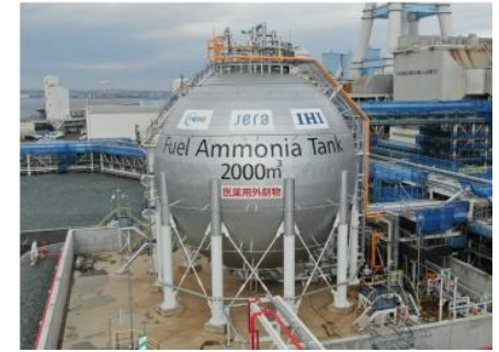
Ammonia Storage Tank
